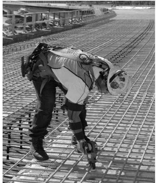
Figure 2. Rebar tying using a MAX-USA RB-392 power tool. Note the bent posture.
