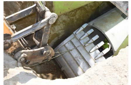
View into the trench where the victim was standing and where the bucket detached from the quick coupler in Case Study #3. [Note – chain placed on equipment post-incident]. Photo: CA FACE program
