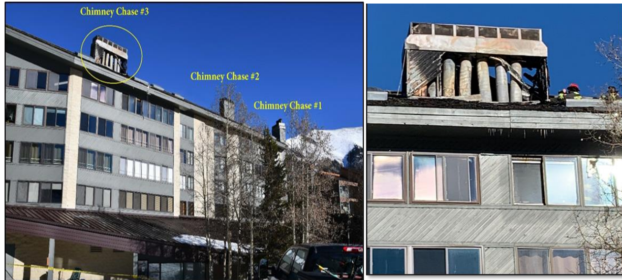
Photo 4 and 5. Left photo shows three of the building's four chimney chases. The fire occurred in the circled 3 rd chase. The right photo is a close-up of chimney chase #3 with the fire damage. The 3 rd chase contained eight flues from the units below. (Both photos courtesy of the fire department's origin and cause report.)
