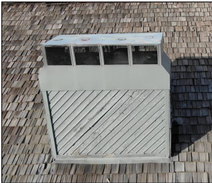
Photo 6. Chimney chase number 2. (Photo courtesy of the fire department's origin and cause report.)
