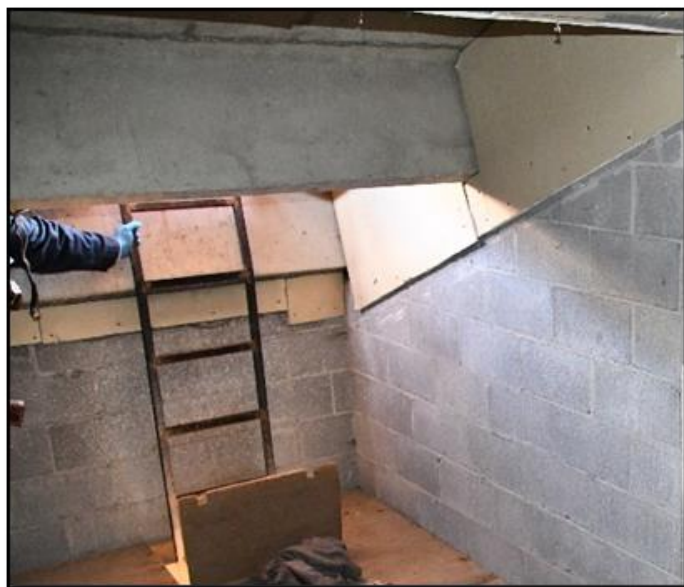
Photo 3. Photograph in the building’s attic. The photo shows a fixed black metal ladder extending from the scuttle-hole on the ceiling of the fourth-floor to the roof access hatch.
